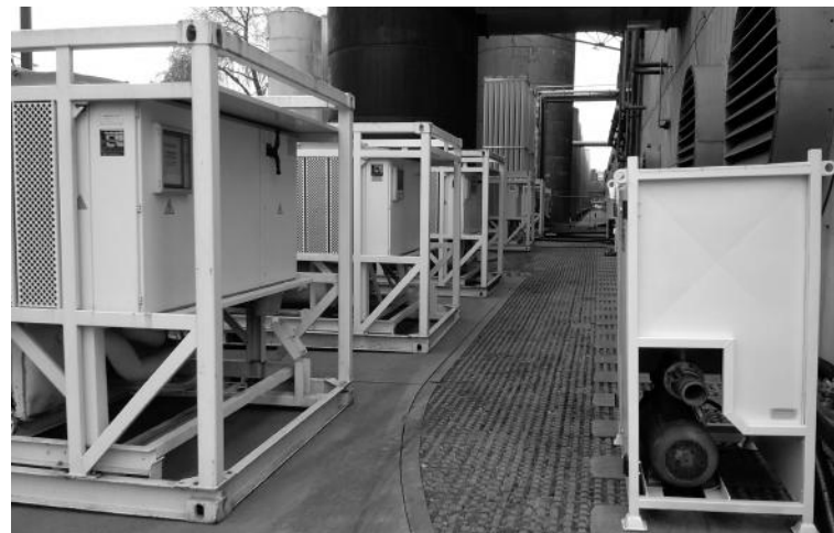
Fig 6: Normal running conditions will have the flow and return temperatures displayed on the controller and the condensing fan motors on top of unit will only run when the unit needs to remove the heat from the condensing coils
