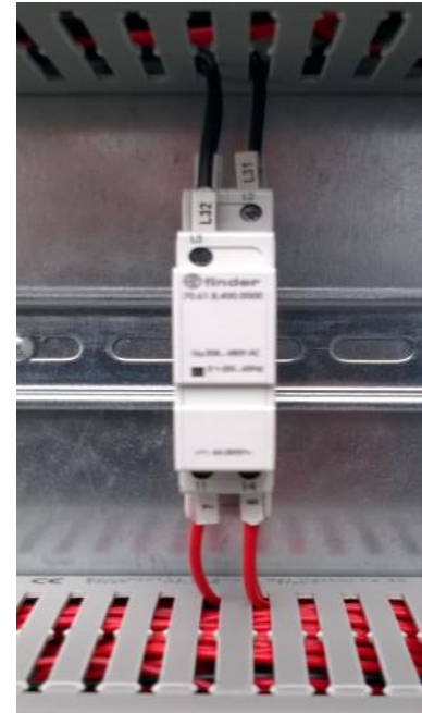
Fig 3 : When the electrical supply is connected and turned on then the phase rotation must be checked inside the electrical panel. Yellow light indicates correct phase rotation.
