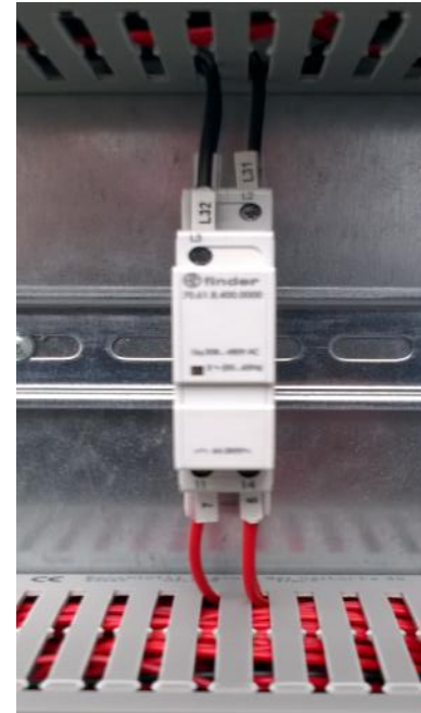
Fig 3 : When the electrical supply is connected and turned on then the phase rotation must be checked inside the electrical panel. Yellow light indicates correct phase rotation.
