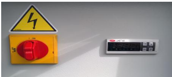
Fig 4: Carel 4 button controller Cooling and Heating is selected through the controller Main isolating switch for power isolation
