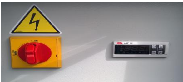
Fig 4: Carel 4 button controller Cooling and Heating is selected through the controller Main isolating switch for power isolation
