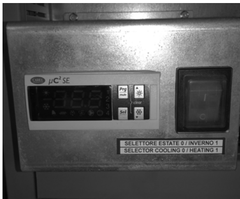
Fig 5: Carel 4 button controller Red switch position 0 Cooling selection Red switch position 1 Heating selection
