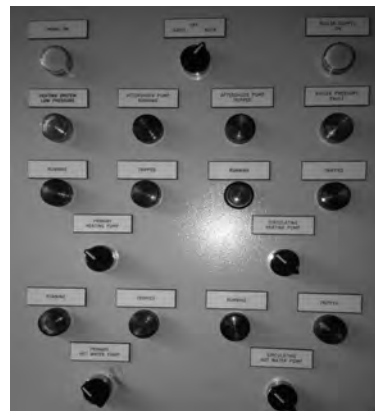
Fig 6: Example of the switch gear control panel
