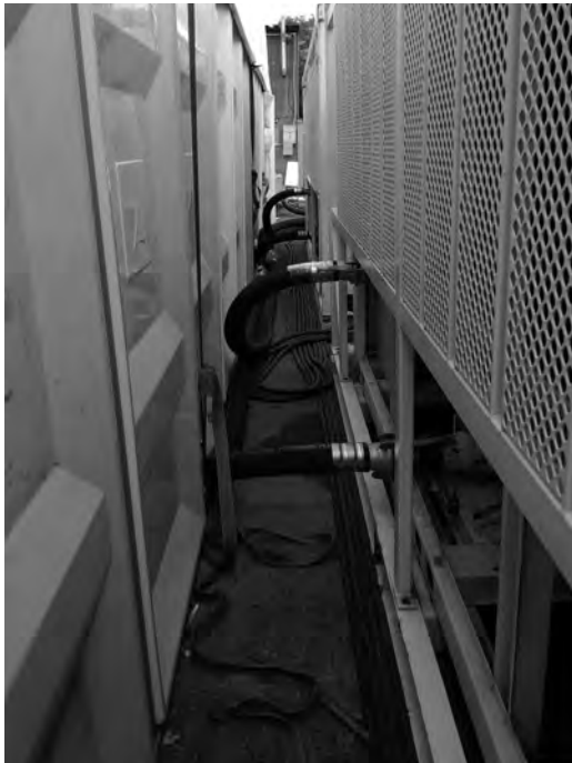
Fig 2 : Return connection at the top of the buffer tank with in line strainer. Flow connection on the outlet of the pump after the heat exchanger
