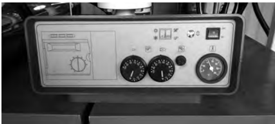
Fig 4: The boiler control panel for the primary side of the boiler
