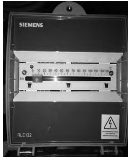
Fig 4: Thermostat used to control Heating and DHW applications. These temperatures can be set independent from each other
