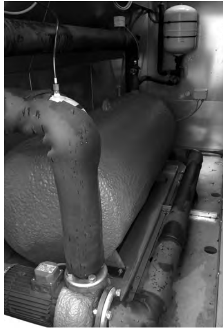
Fig 3: Buffer tank to be used to fill the chiller with water and purge the system of Air
