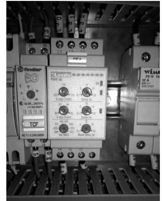
Fig 4: If phase rotation is incorrect then the controller will not light up and the unit will not work
