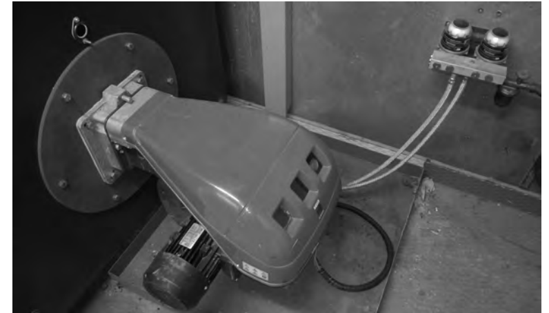
Fig 5 : Gas oil 2 stage burner. Twin tiger loop filter system
