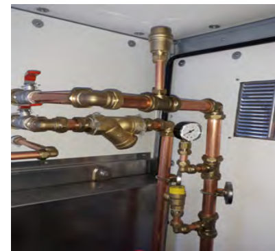
Fig 9 : Flow and return connections inside of the boiler. water filter is on the return connection. Make sure the secondary side of the boiler is filled with water before switching on the secondary pump
